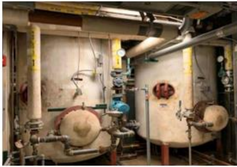
Domestic Water Tanks – corroded & leaking
