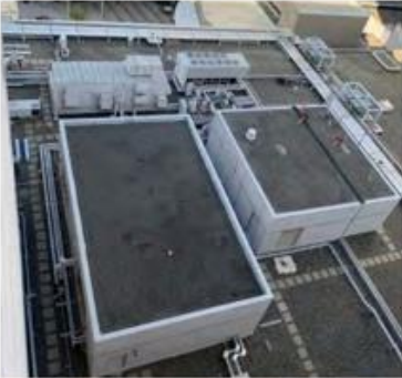
Building Exterior & Roof Failures/leaks
