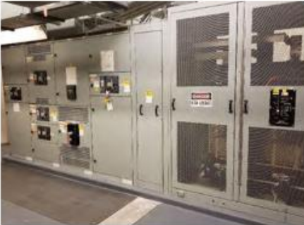
Emergency Power ATS units – end of life
