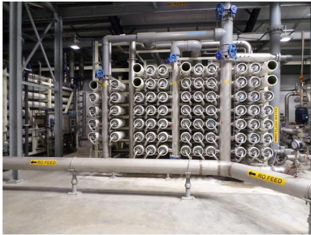
Existing RO System
